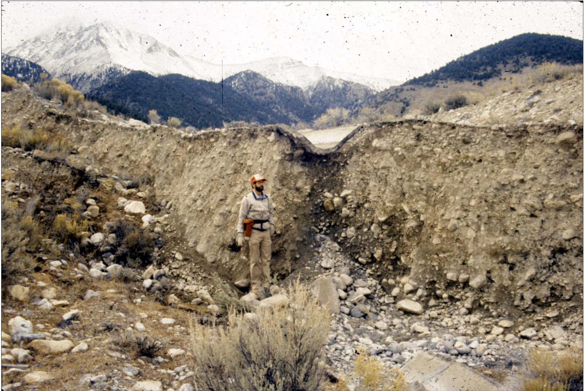
Damaged irrigation ditch at Rock Creek after Borah peak quake.
