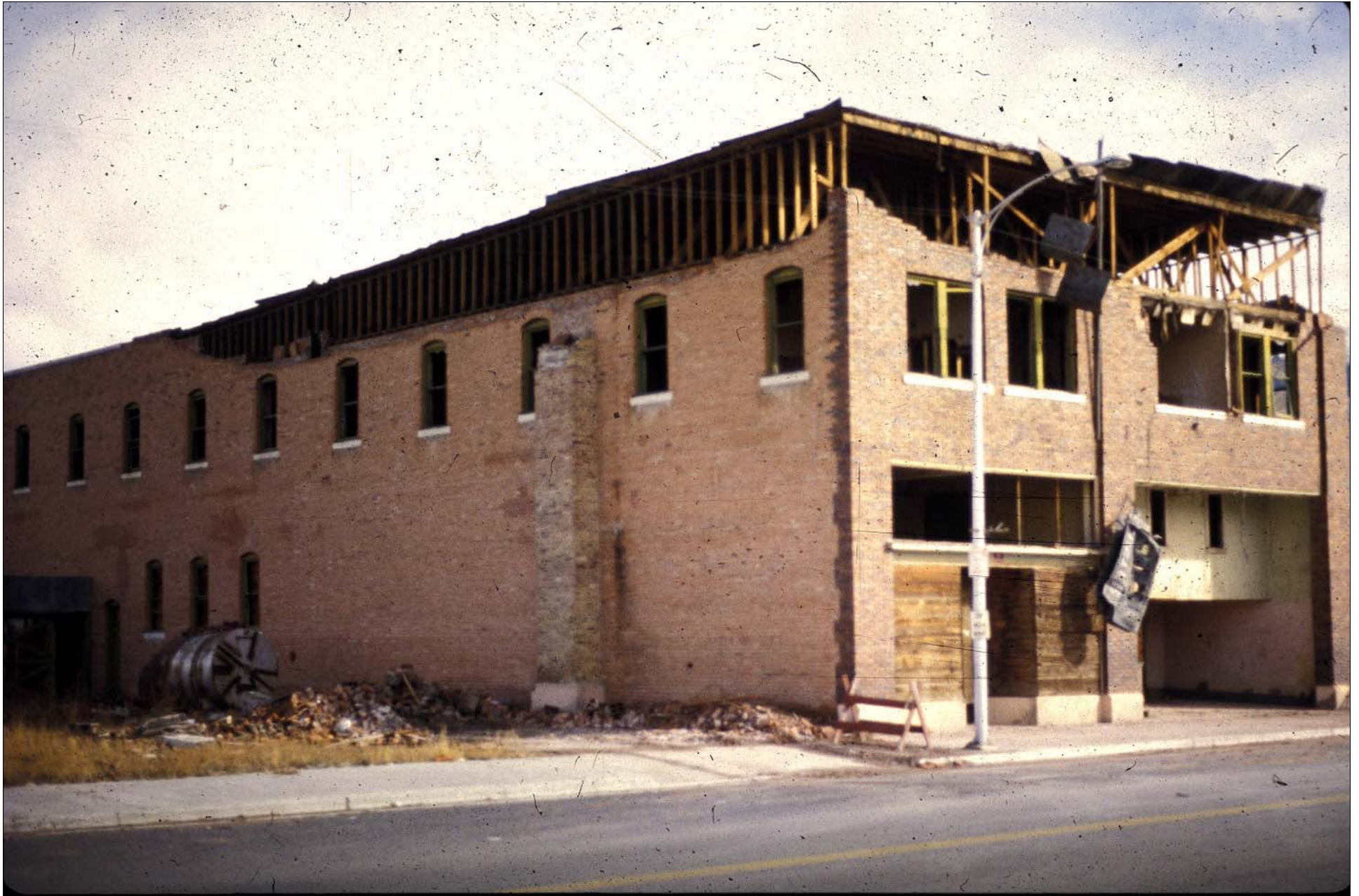
Old brick building which was damaged by shaking of Borah Peak earthquake.
